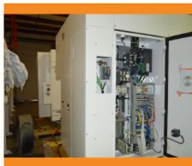
Inside Electrical Cabinet
